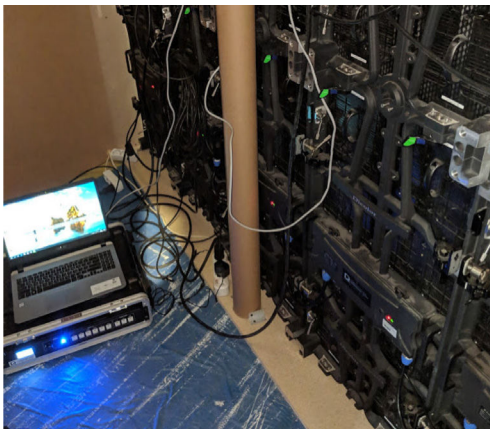
Bad example of using cardboard tube for securing a screen installation.
