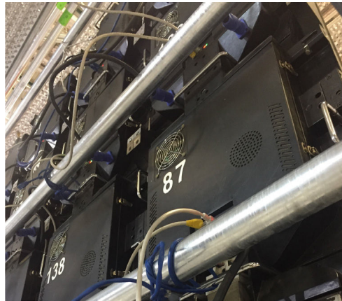
Bad example of using ethernet cable to secure an installation
